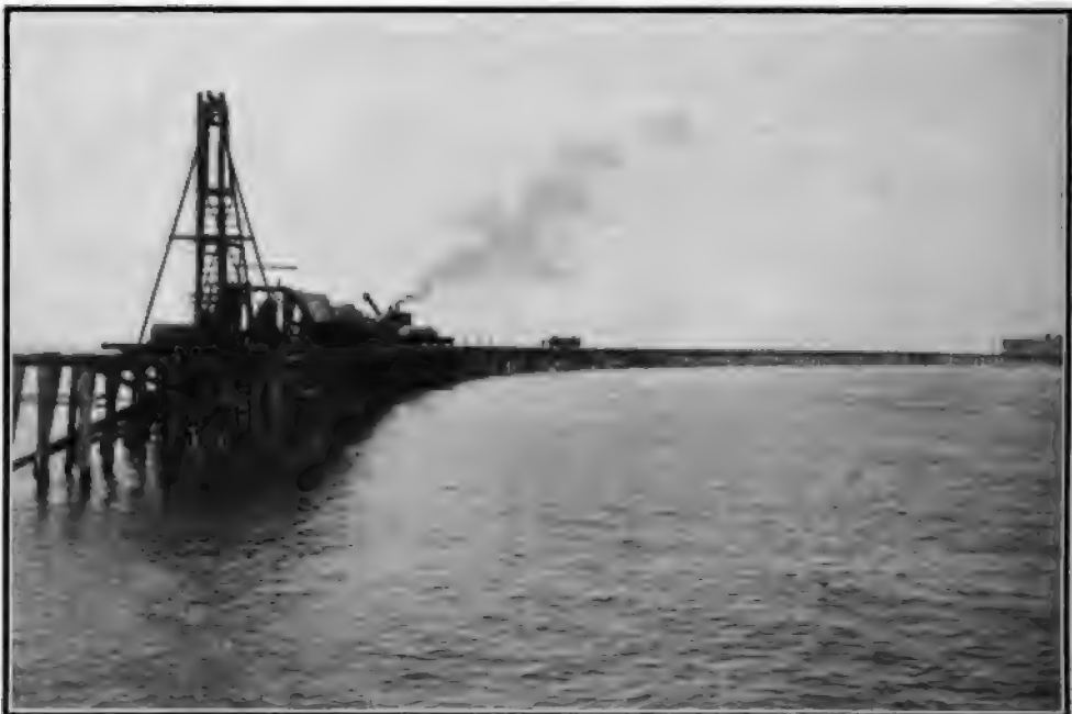
The trestle was built by piles and a pile-driver is the advance guard of the work
